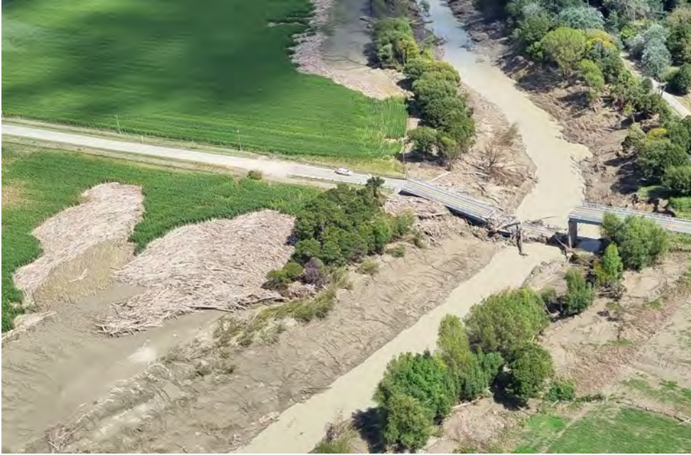
Figure 4: Broken State Highway 35 at Hikuwai
